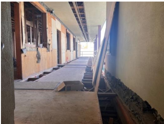
Raising the deck to meet the door entry on the second floor
